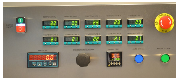
Control panel showing ten temperature controllers, plus digital pressure and digital dwell time controllers.
